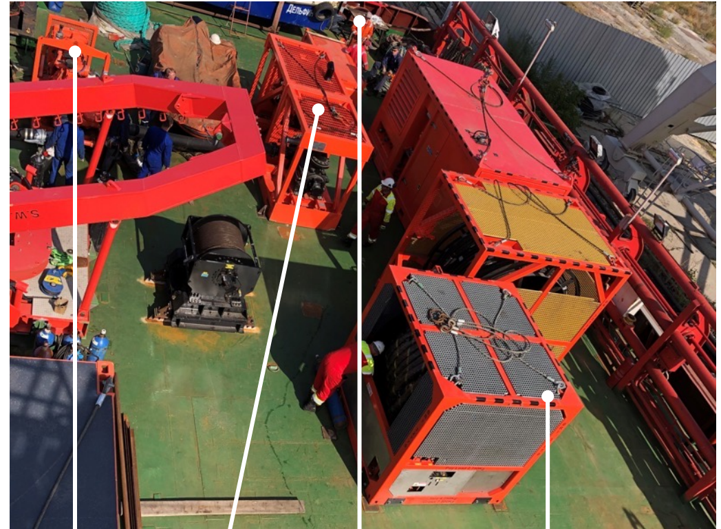
Water Lift Pump
